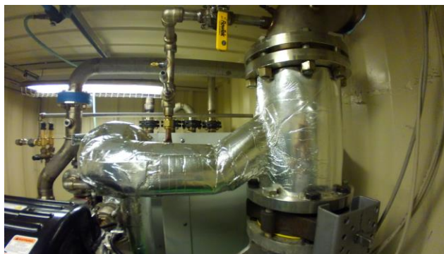
Figure 6 Lagging installed on pipe
