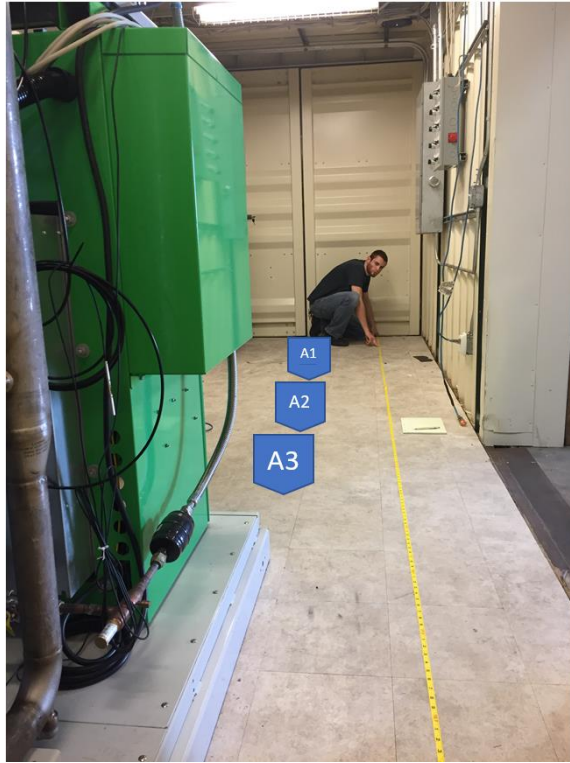
Figure 2. View from inside the ORC shipping container
