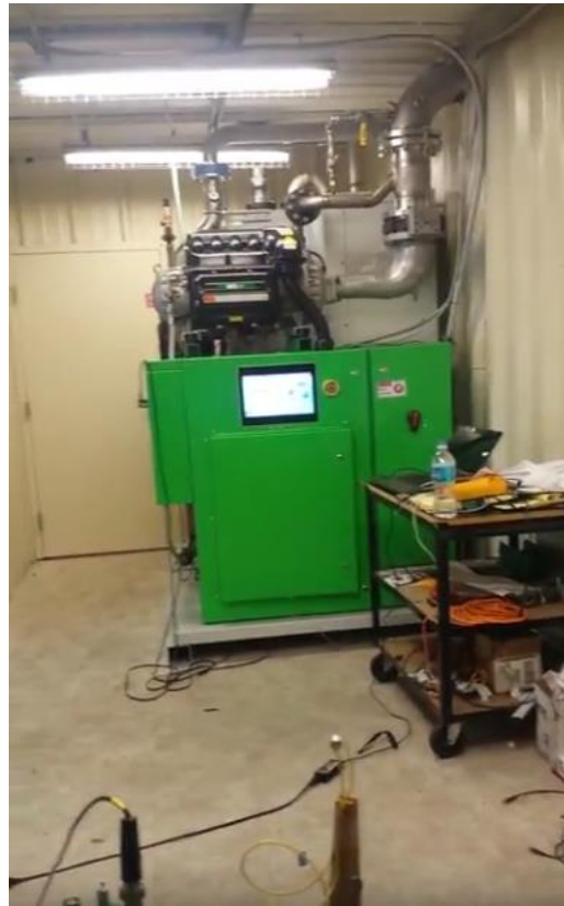
Figure 18. ORC system positioned in shipping container
