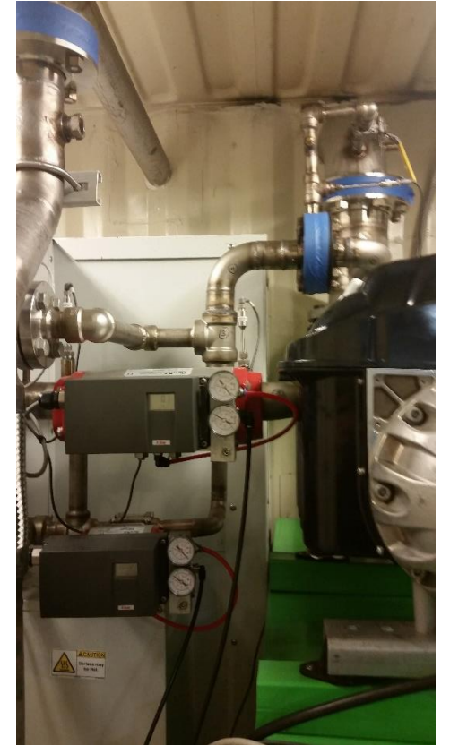
ORC Turbine Bypass Line
