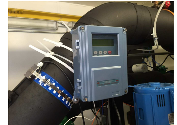
Installed & Mounted Sensor Module
