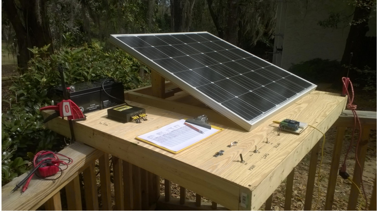
Figure 34. Power System Test Setup.
