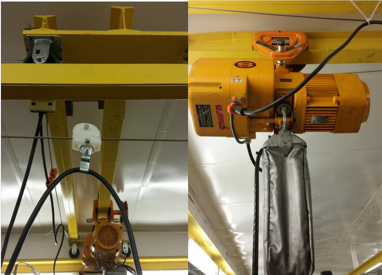
FIGURE 2 - THE CURRENT GANTRY (LEFT) AND POWERED CHAIN HOIST IN USE (RIGHT)
