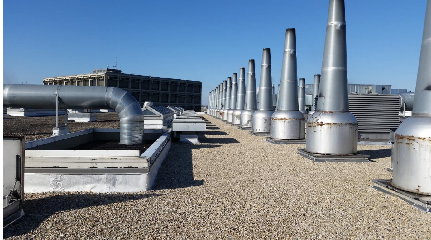
Figure 3 – CTC Exhaust Vents
